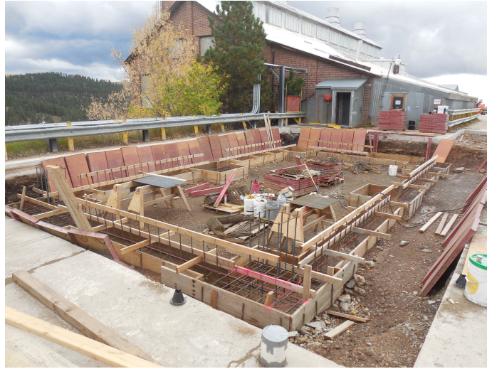
Figure 10.1.3: A picture (October 2016) of the additional building being constructed to house the radon-removal system (RRS).
